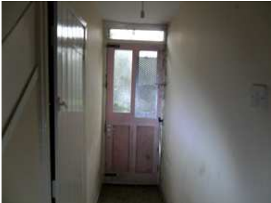
Photo: 32 Rear Door need replacing
