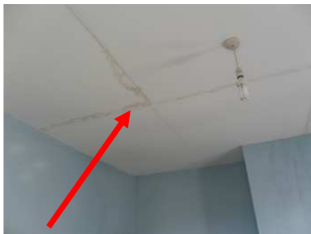
Photo: 21 Water tracking back to ceiling
