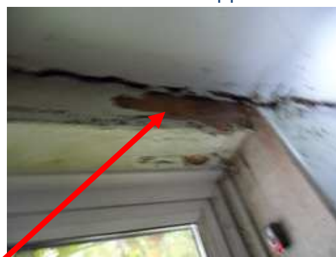
Photo: 17 Localise damp to the wall.
