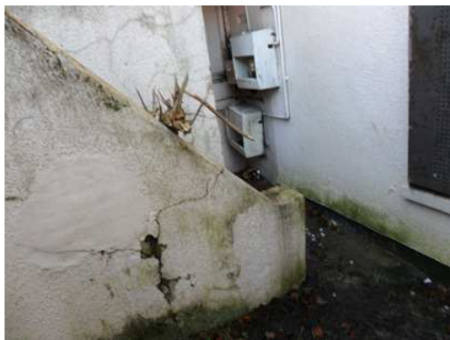
Photo: 12 Front garden wall failure
