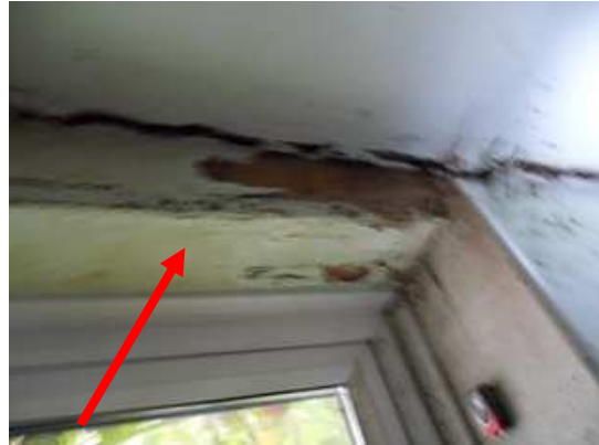
27 Damp in the wall
