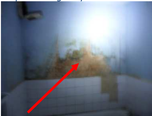
Photo: 16 Localise damp to the bathroom wall.
