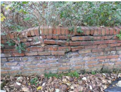
Photo: 13 Rear garden wall failure
