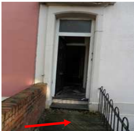
Photo: 33 Defective areas of the slab
