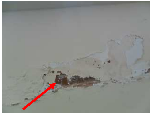
Photo: 29 Damp in the wall
