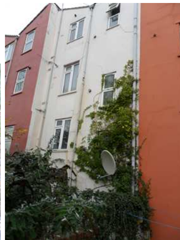
Photo: 14 Rear elevation wall failure
