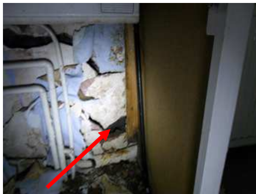
Photo: 28 Damp in the cupboard wall
