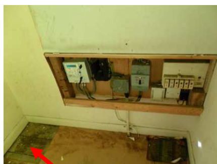
Photo: 23 water stained floor board
