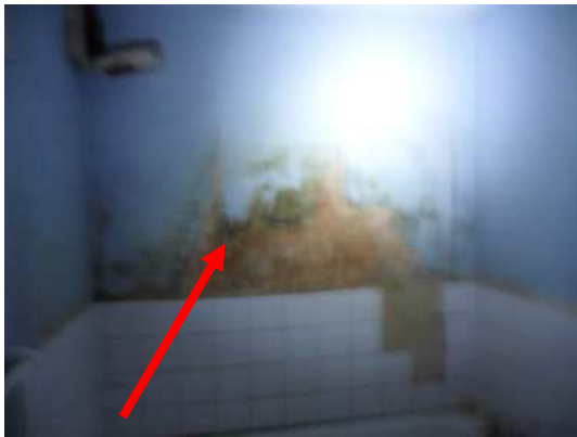
Photo: 26 Damp in the bath room wall
