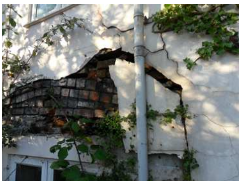
Photo: 10 Lintel failure
