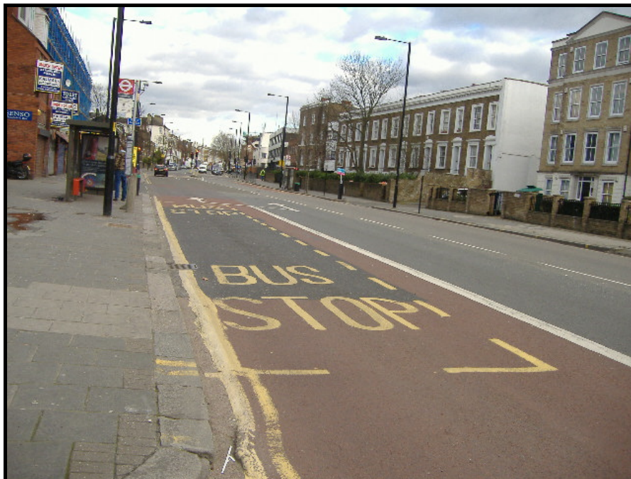
Figure 2.1 – View of the Missing Red Surface within the Bus Cage
