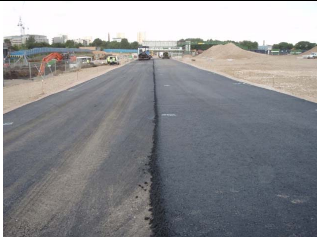
Another section of internal haul road is tarmaced. Currently 8km of internal haul road is tarmaced. Other areas are covered with the human health protection layer (hardcore) as soon as final levels are achieved. Prior to that they are dampened down using mobile bowzers.
