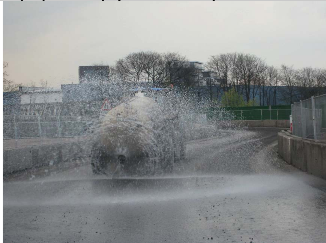
One of 10 mobile bowers on site that constantly dampen down the site roads
