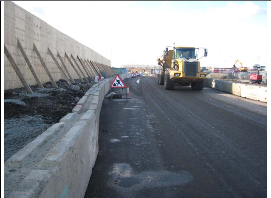
Main haul routes hard-surfaced for easier dust management. Strict speed limits (reduced further in May from 20 to 15 mph) help reduce dust being generated
